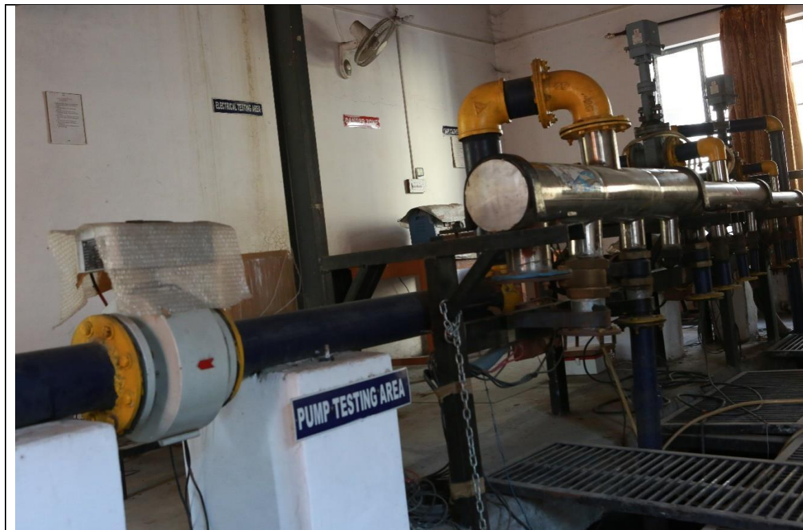
Fig.4: Pump Testing Area
