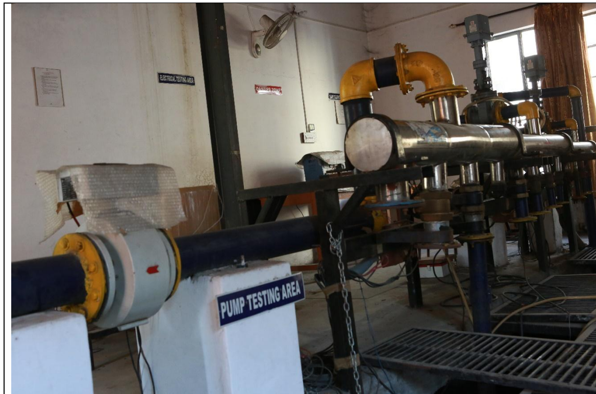
Fig. 5: Pump Testing Area
